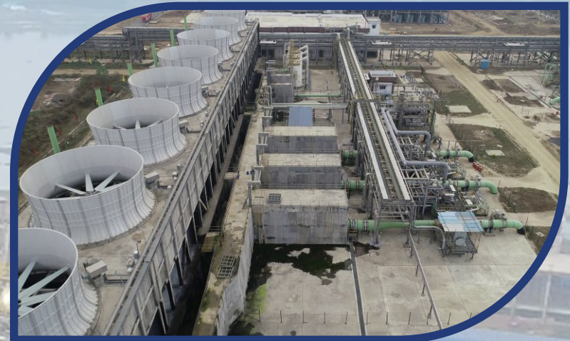
Ammonia Cooling Tower
